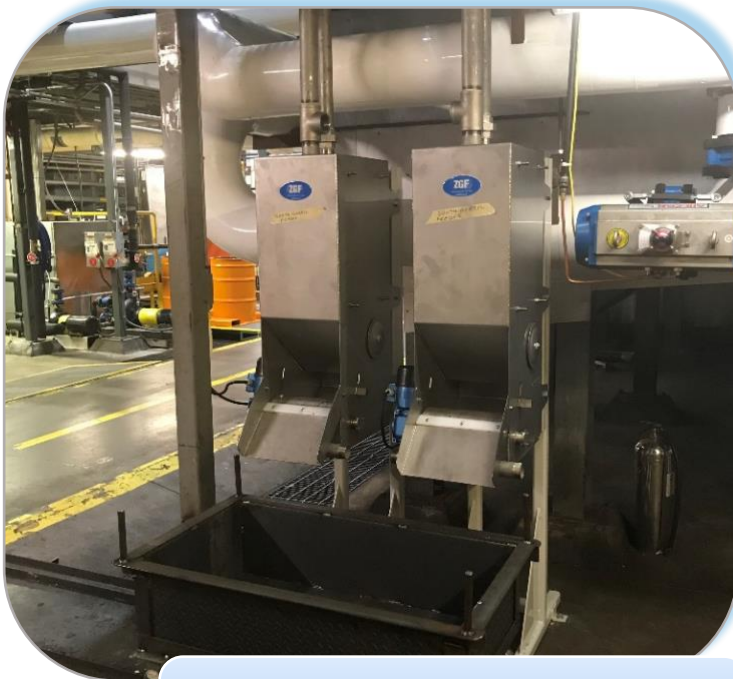
Weld Balls and Metal Fines Captured by Maggie and Removed by SD+
