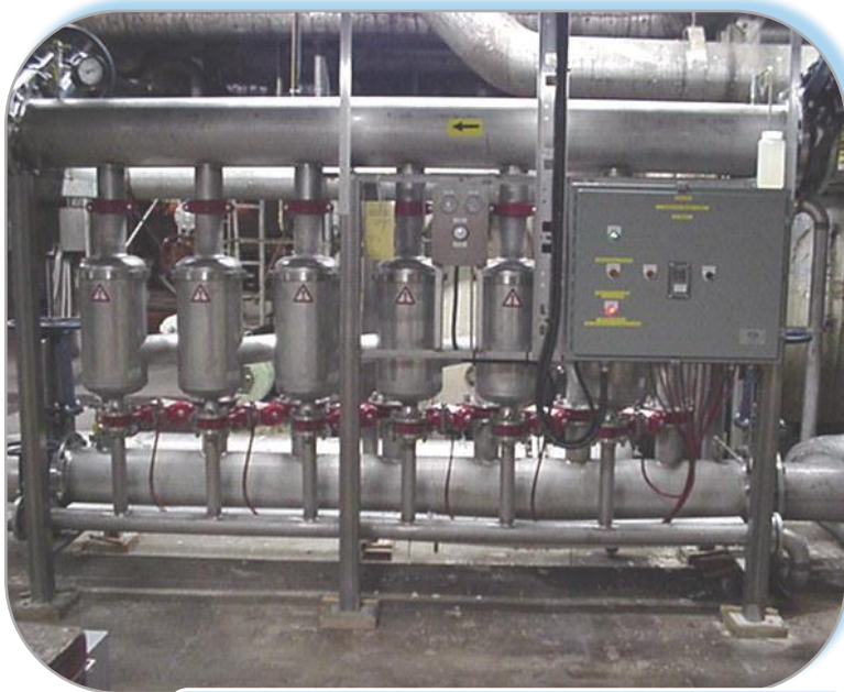
EZ Clean EC700S Filtration System
