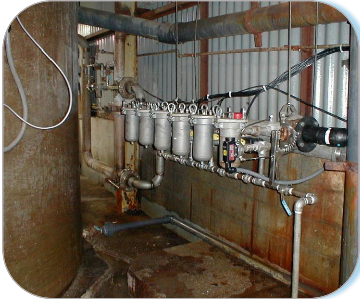
ZGF EZ Clean EC100S, 6-Pod 316 stainless steel pods / piping Design: 150 gpm @ 210 psi
