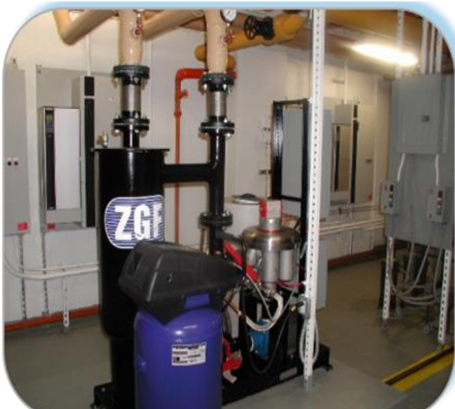
Phoenix Forced Sedimentation Filtration System (FSFS) installed on the condenser closed loop to remove suspended solids
