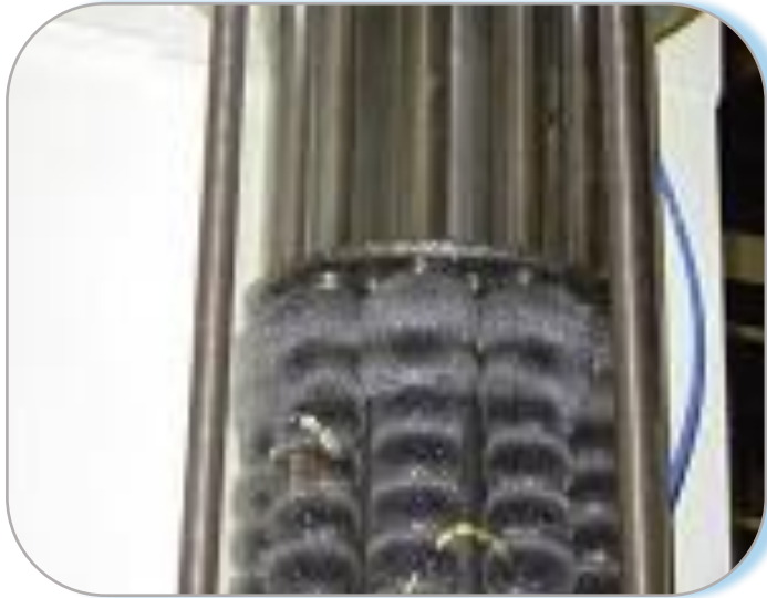
Internal view of Maggie prior to purge to remove contaminants
