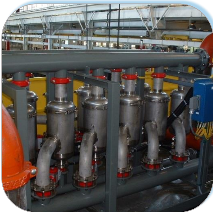
ZGF EZ Clean EC700S, 6-Pod Automatic, Permanent Media Filtration System, design flowrate of 600 gpm
